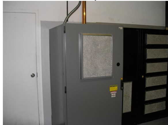
Not much to it – AC in and RF out (the rest of the signals enter via the floor trough below)
