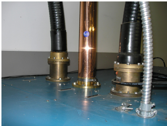
The shiny one is the new transmission line for the NX50
