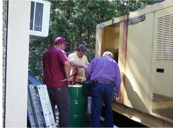
Refueling the WYDE-FM gen from a 55-gallon drum
