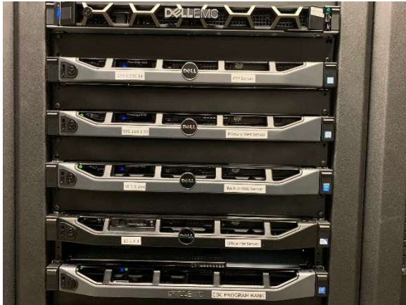
Figure 1 -- The server stack in Denver. The primary web server is third from the top, a hot-rod Dell PowerEdge R430 that we installed last fall.
