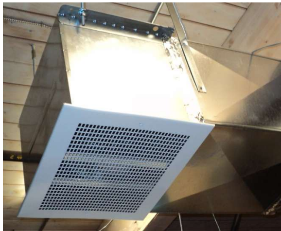
New exhaust system at KKPZ.
